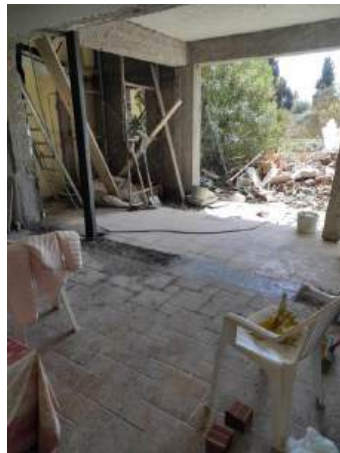
This used to be a nice lounge
