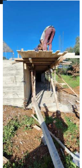
Water storage moving outside
