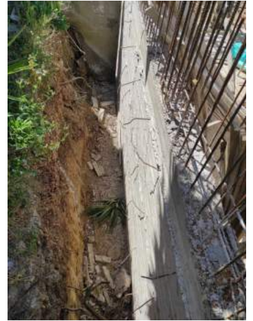
Needs tanking first
