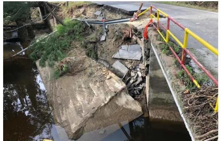
Afra bridge is falling down
