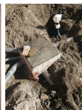
New drainage confluence for three buildings
