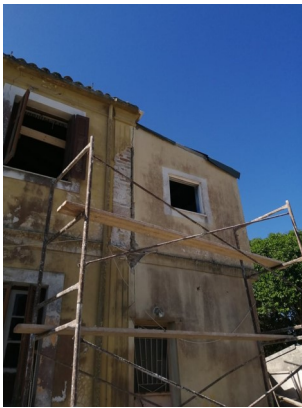
Two parts of this building were separating
