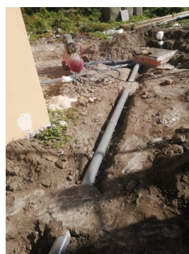
Pipework is always photographed so we know where it is
