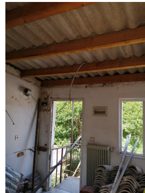
Roof tiles off
