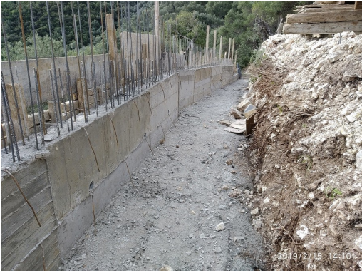
It must not slide or crack
